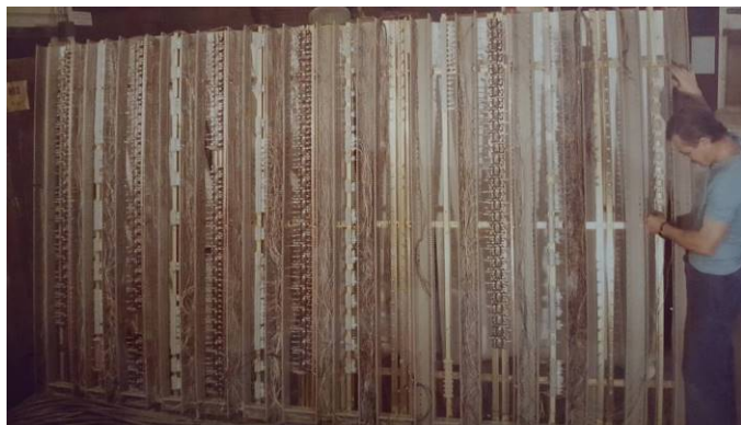
Bornier " raccordement mesures " RAM (partiel)
